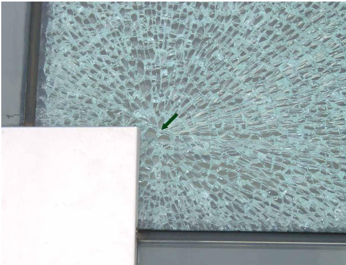
A characteristic “spontaneous” fracture pattern in a toughened glass window. The nickel sulphide inclusion is found at the initiation of failure (at the centre of the butterfly pattern, arrowed)
